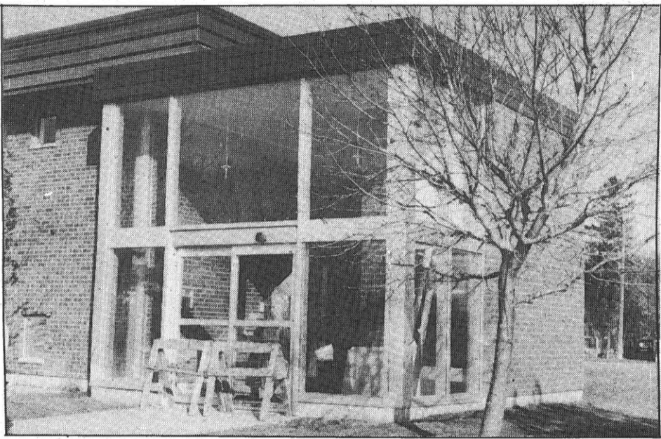
The addition that will house the hydraulic lift and enclose the stairs at the Millbrook Medical Centre is near completion.
